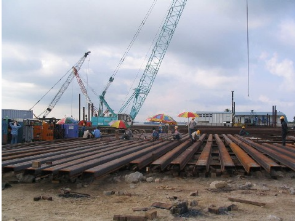
Sheet pile fabrication yard - to join 2 pieces of sheet piles (12m, 14m, 16m) by butt welding and splice plate
