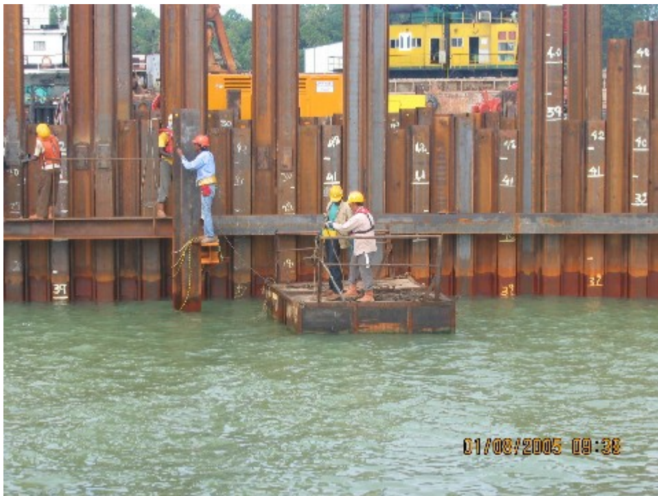
Sheet pile installation pattern - alternate pitching and driving (neighbouring welding splice staggered)
